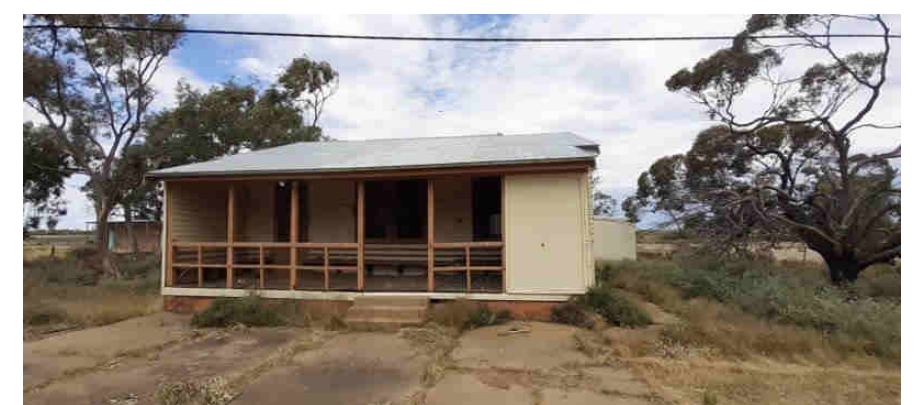
Old school building (derelict/unsafe).
